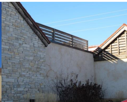
Unique design elements that also provide attractive screening for equipment.
