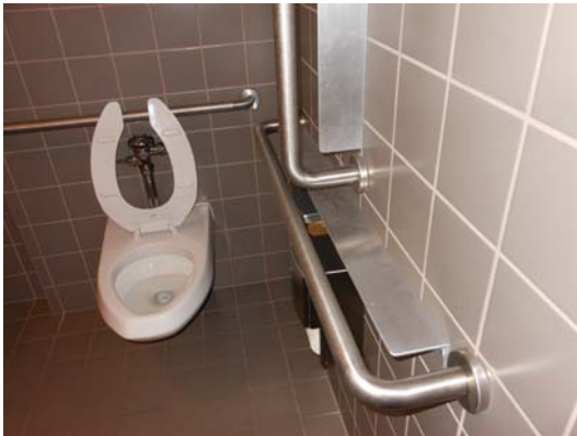
Photo 4: Replace the grab bars with a style that is 1 1/2" from the wall (currently 4") in the 2nd floor men's toilet room and family toilet room.
