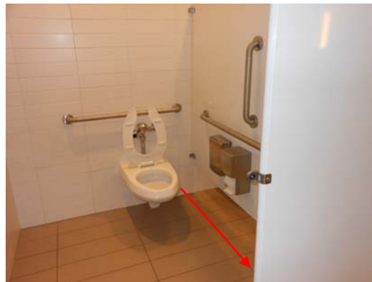
Photo 5: Modify to provide 48" in front of the toilet in the women's toilet rooms (currently provides 45").
